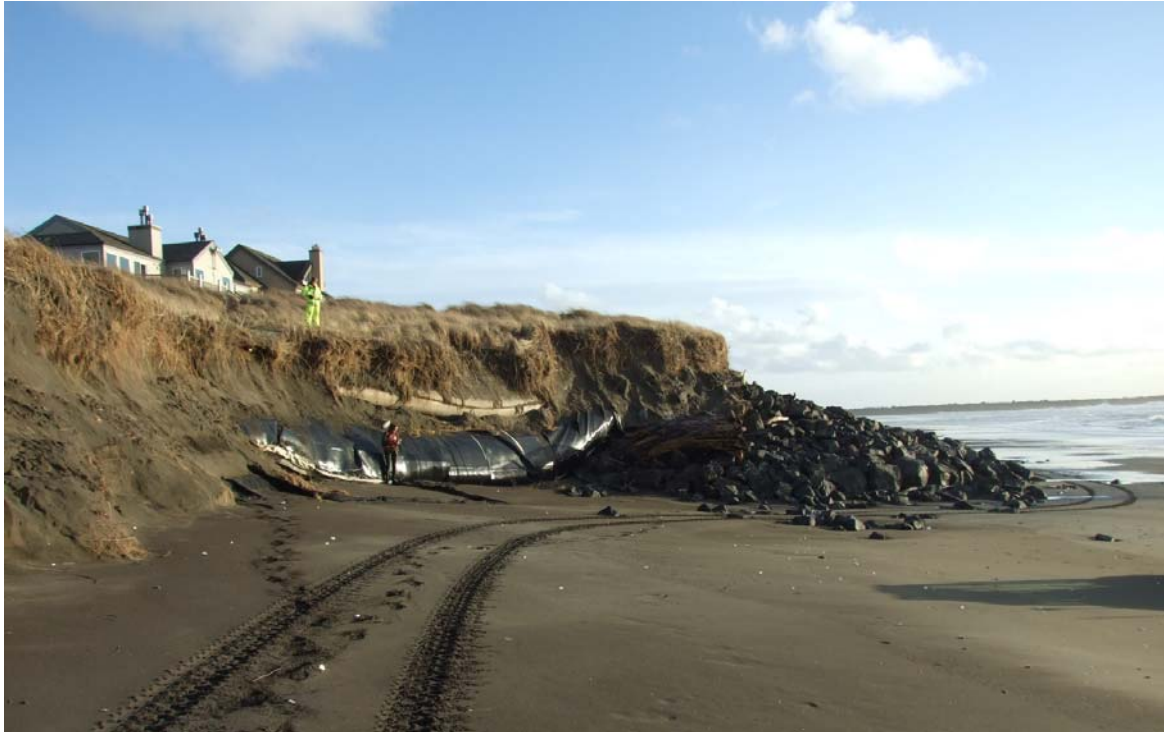
Figure 7. Dune erosion at Ocean Shores during winter 2010/2011 further exposed the rock revetment and geotubes that had been installed in 1996 and 1998 to protect condominiums and houses along this vulnerable shoreline reach.
