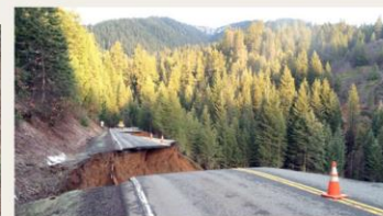
March 16: Northern California highway crumbles as storm-soaked hillside collapses. Highway 3 near Rush Creek Road just north of Weaverville in Trinity County. Photo: LA Times
